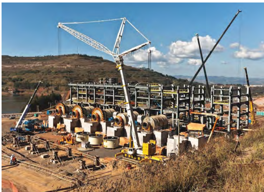
Vale, the leading iron ore producer, accounted for almost 17% of world iron ore output last year. Pictured here is construction of Vale's newest iron ore beneficiation plant, located in the Itabira region of Brazil. (Photo courtesy of Vale)
