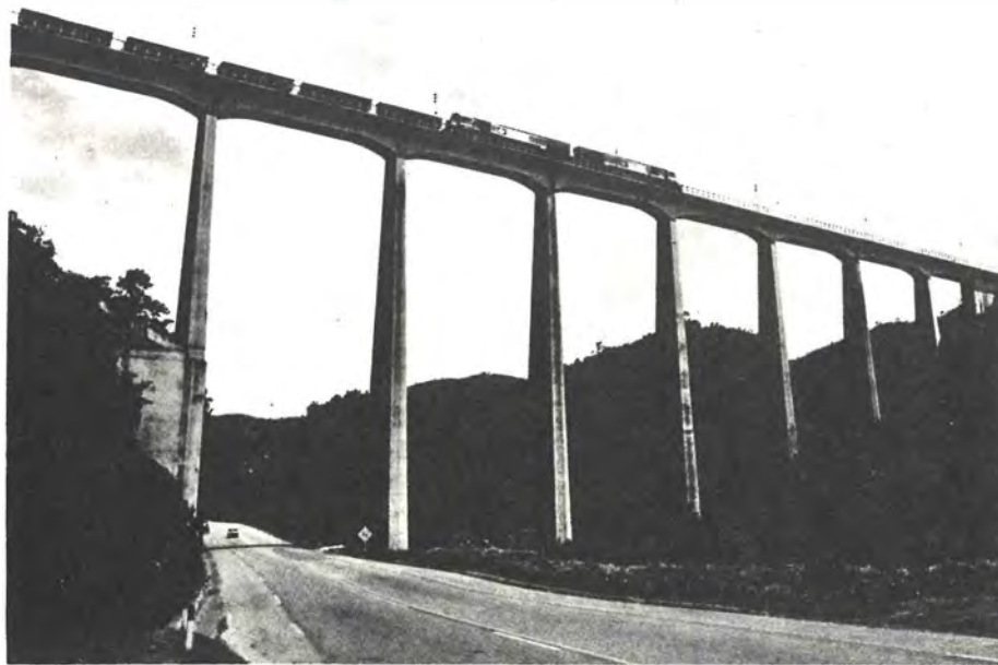
The Funil overpass, located at km 72 of the Fabrica branch line of EFVM, is 92 meters high. CVRD plans to invest 300 million dollars to electrify EFVM during 1982/83.
